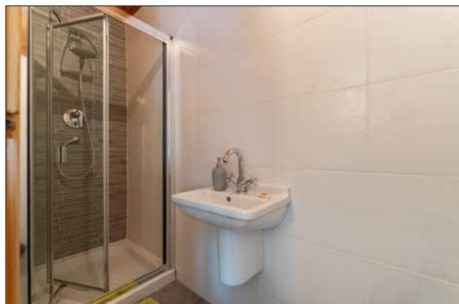
ENSUITE SHOWER ROOM: Low flush WC, wash hand basin, tiled shower enclosure, tiled floor, fully tiled walls, tongue and groove panelled ceiling.
