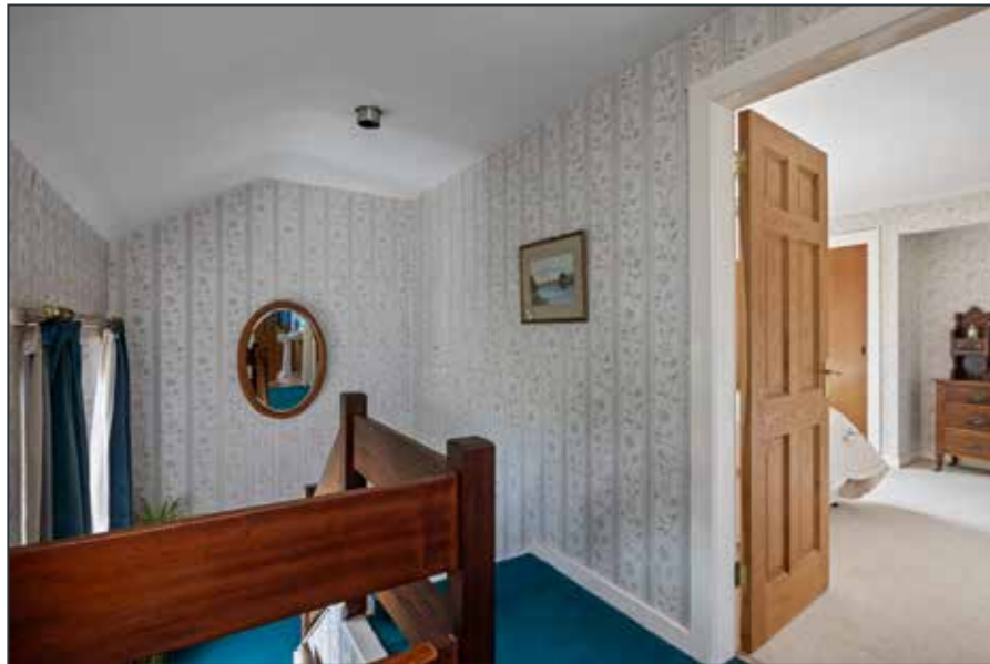
FIRST FLOOR LANDING: Storage cupboard, linen cupboard with shelving and gas boiler.
